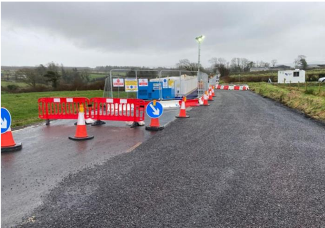
Figure 2-11: Operational Joint Bay with Passing Bay (on the Kilpaddoge Knockanure 220kV UGC Project, Co. Kerry)
